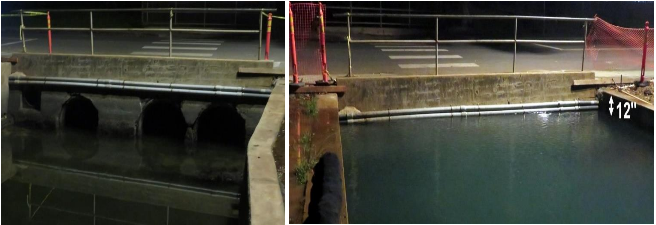
Photo 6 – 9:35 pm 0.05-ft. low tide (0.33) Kewalo Harbor culverts. Photo 7 - Dec. 5, 4:41 am 3.22-ft. (2.65) King High Tide. The water rose within about 12” of the top of the canal side banks and 16” of the Ala Moana Park Drive street level.
